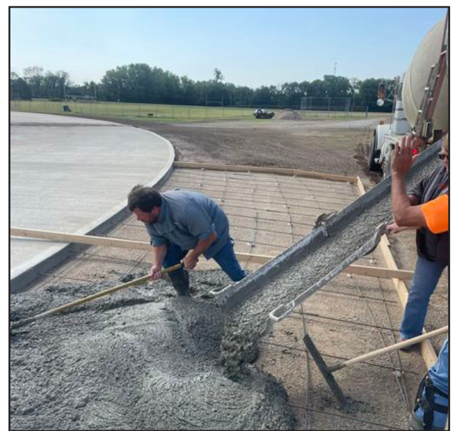
TRACK RENOVATION AT JIM METTNER FIELD MAKING PROGRESS. Fisher Tracks began construction of the new track on June 24. (Courtesy Photo)
